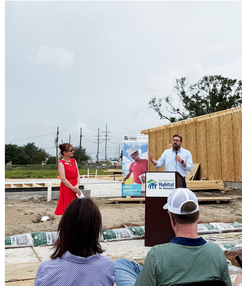
Construction underway for homes in the Rising Oaks community in Terrytown, Louisiana.
